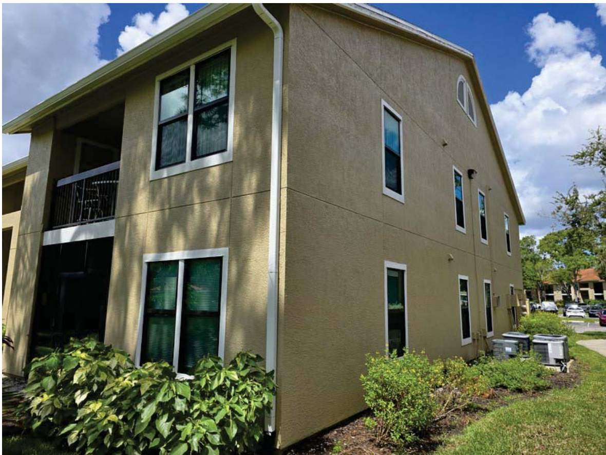
BUILDING'S OLDER SLIDING GLASS DOORS WERE NOT IMPACT RATED
