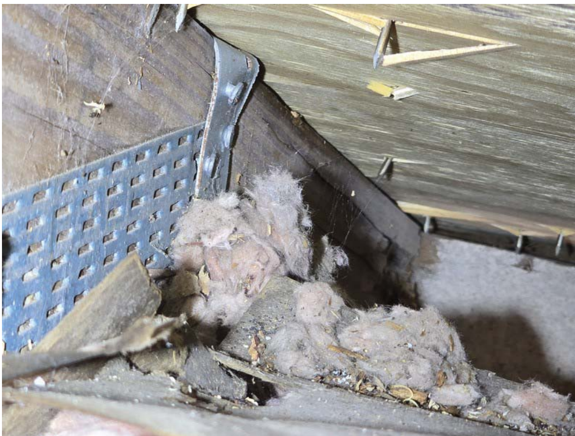
ROOF TO WALL - STRAPS FRONT SIDE - OK
